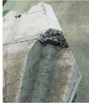
Figure 6.2 - Local rupture on a (concrete) droxel [40]
