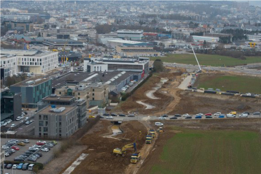
Fig 2: Photograph of the Ban de Gasperich in 2018. The Weierbach ecological couloir under construction. Photothèque Ville de Luxembourg.
