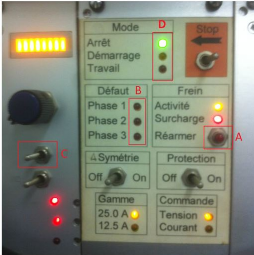
Figure A.7: Zoom of the left inverter panel (taken from the lab user guide made by Messr. Chevalier and Templier)
