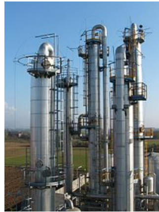
FIGURE 2.2 – Colonnes de distillation industrielles
