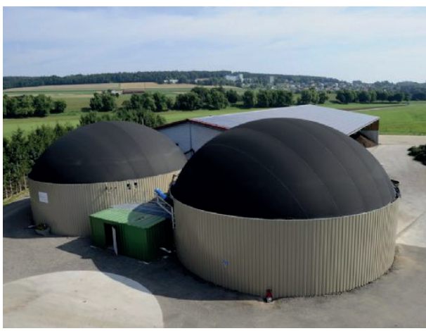
CENTRALE BIOGAZ BARDAGE BOIS Jura - France
