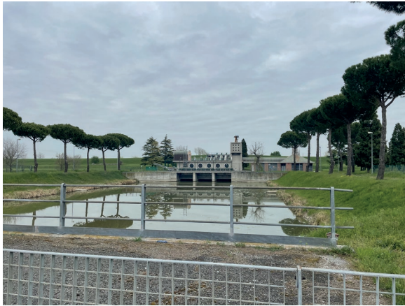
Fig.26 Station de pompage, province de Padoue
