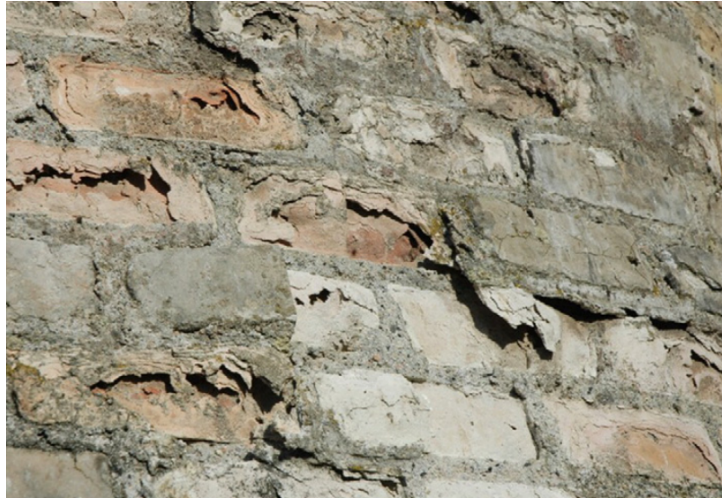
(a) Flaking of the masonry.
