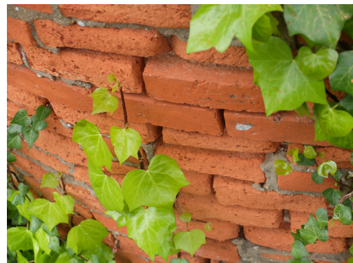
(b) Missing joint mortar.
