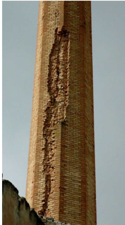
(c) Cracks due to lightning strikes.
