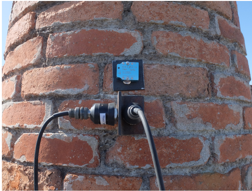
Figure 3.16: Mounting of the accelerometers on the chimney.
