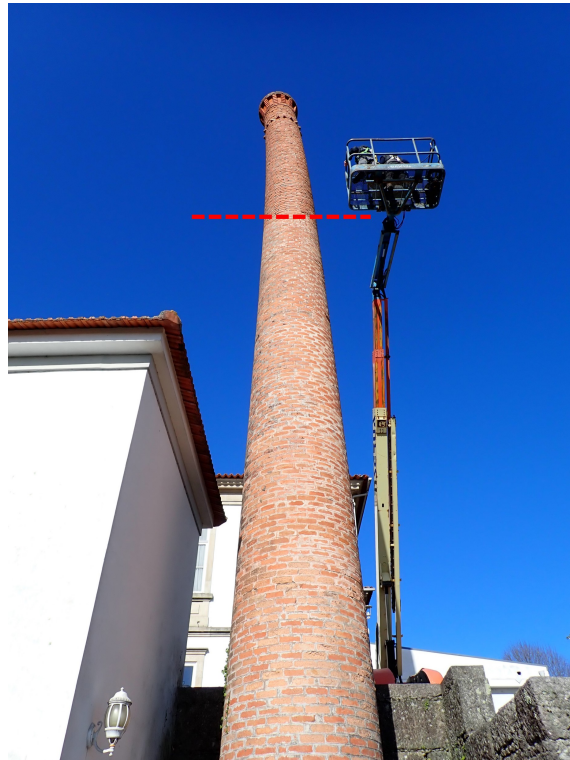
Figure 3.13: Demarcation between the bricks of two different colors.
