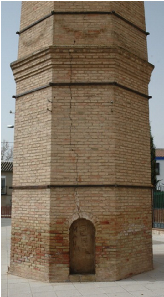
(b) Cracks due to temperature gradients.
