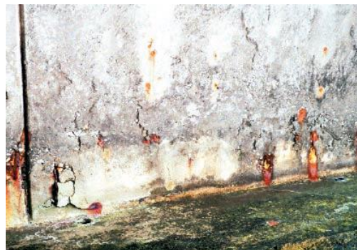
Figure 18: Piqûres de corrosion
