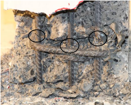
Figure 98 - Rupture des armatures colonne C3C
