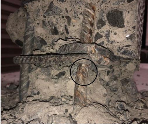
Figure 92 - Rupture des armatures colonne C3A
