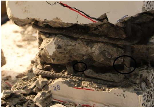
Figure 83 - Rupture des armatures colonne C2B
