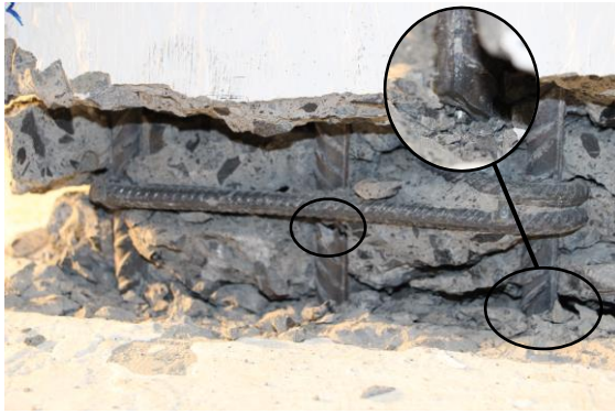
Figure 72 - Rupture des armatures colonne C1A
