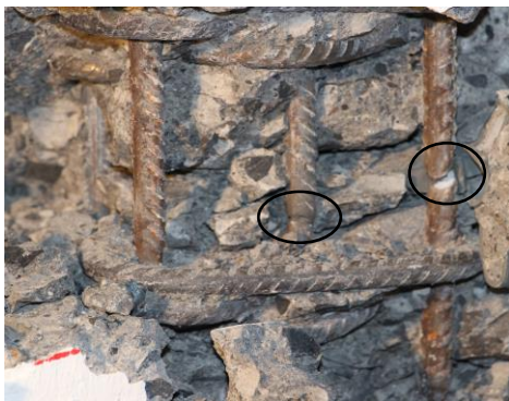
Figure 95 - Rupture des armatures colonnes C3B
