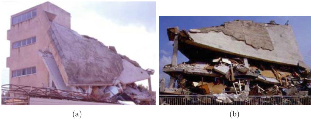
Figure 1.2: Collapse after the earthquake in Athens in 1999, source [4]
