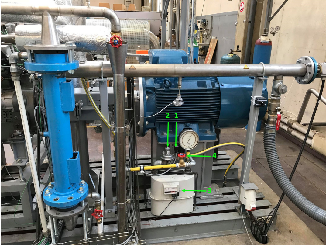
Figure 2.3: Natural gas pipe devices: (1) emergency stop valve, (2) zero pressure regulator, (3) Krom schroder gas meter, (4) slide valve.
