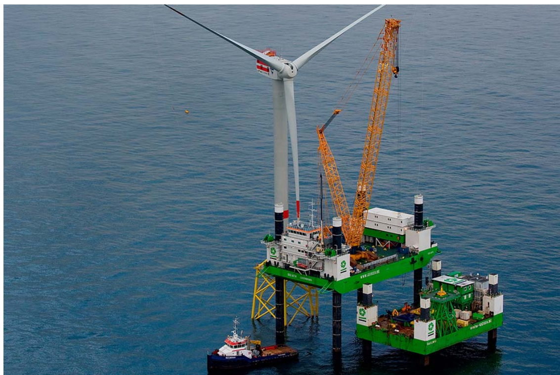
Figure A3.1: Picture of the assembly of an offshore GE Haliade 150 6MW in the Merkur wind farm in North Sea
