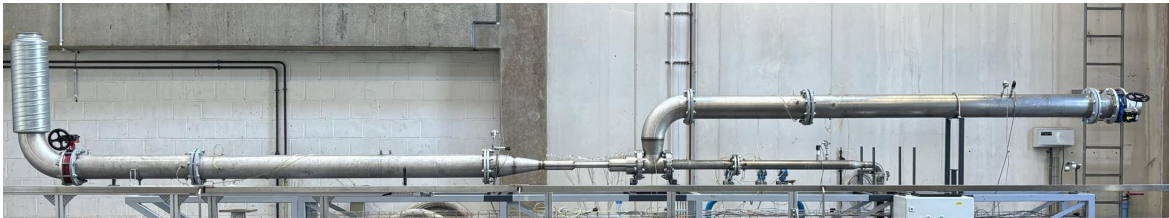
Figure A.1: Picture of the complete installation
