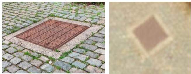
Figure 20. Field images and snapshots from orthophoto – Metal drain top
