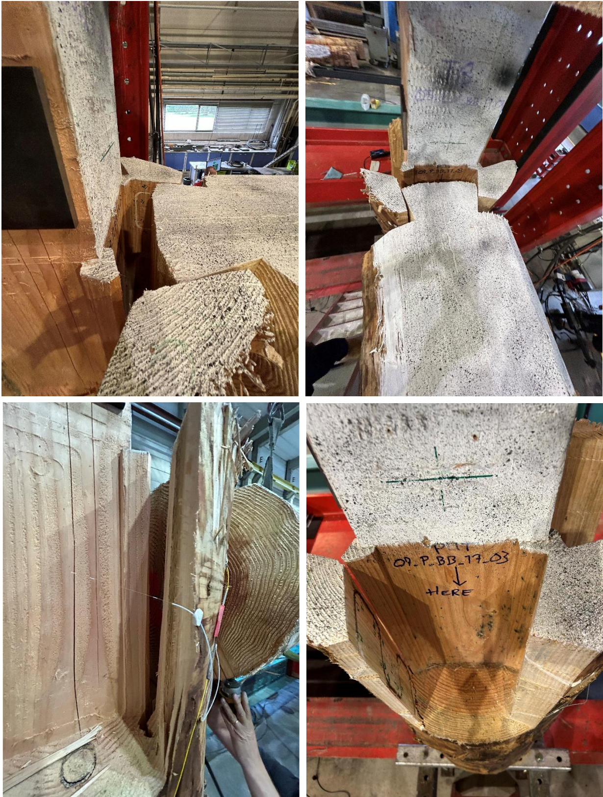
Figure 66: Views of the cracks observed on the column. Source : Serena Van Nimwegen.
