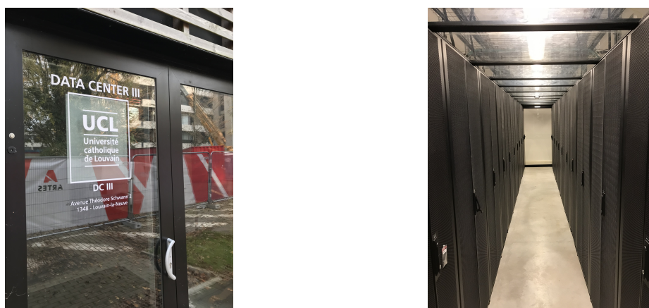
Figure 1.1: Photos taken during the visit of Data Center III at the UCLouvain [5].
