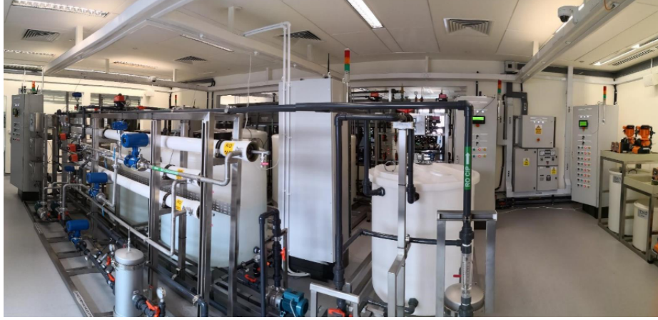
Figure 1.1: Picture of the SWaT System in Singapore [6]
