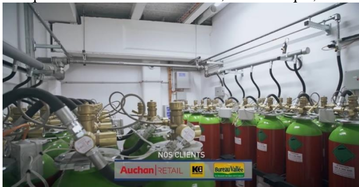
Photo 6 : salle incendie (Comarch France, 2018)
